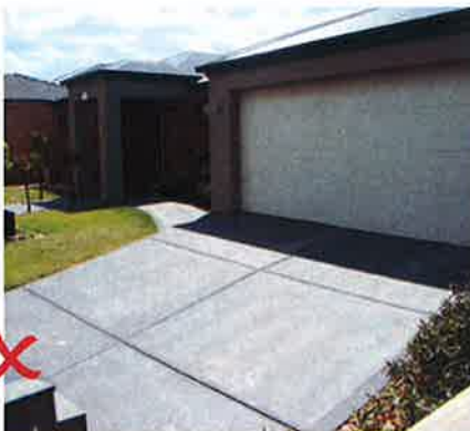
Example of non compliant driveway, plain concrete not permitted.
