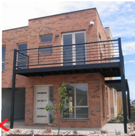
Example of non compliant materials treatment, no differentiating materials.
