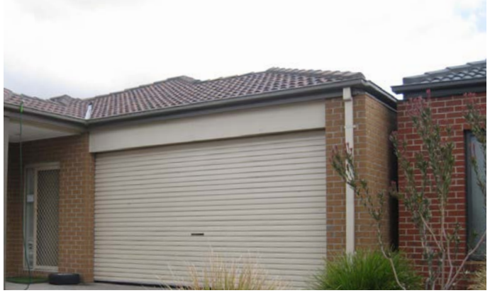
Example of infill panel above opening not permitted
