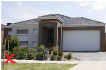
Example of non compliant treatment no eaves
