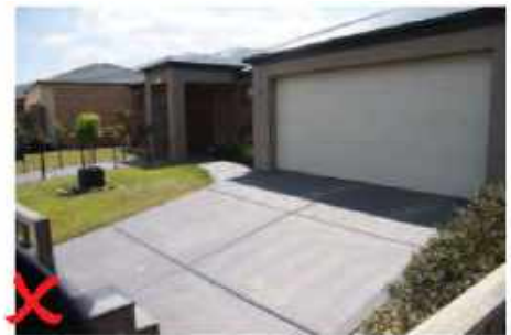
Example of non compliant driveway, plain concrete not permitted.
