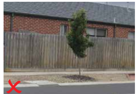
Example of non compliant timber paling fence without capping and exposed posts
