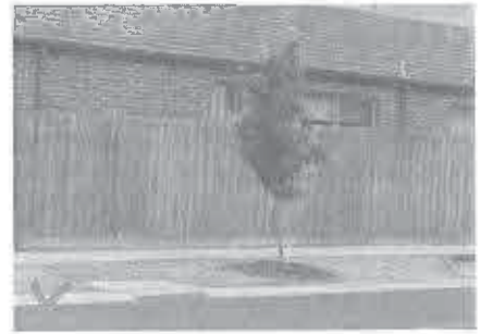
Example of non compliant timber paling fence without capping and exposed posts
