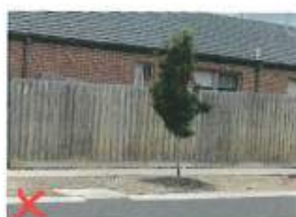
Example of non compliant timber paling fence without capping and exposed posts.
